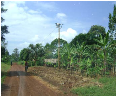
Electricity grid extension to Naminya Resettlement
