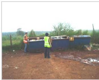
Waste skips for different categories of waste at the dam site
